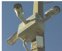
Urban Witness Field Deployed CCTV System
